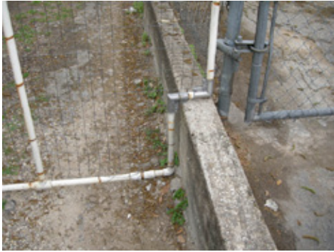
This pvc pipe gate was carefully made to fit the existing wall. Though constructed of inexpensive materials, the planning involved reveals this is not just a temporary fix.
